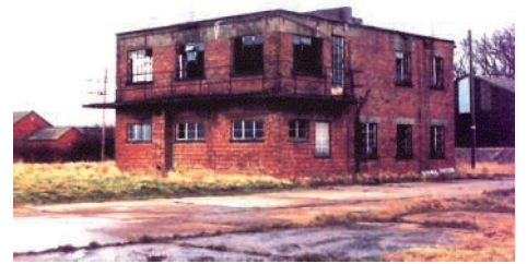
The Thurleigh Control Tower showing the deteriorating condition towards the end of the 20th century, before it was torn down.
